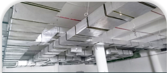
AC DUCTING AND FRESH AIR
