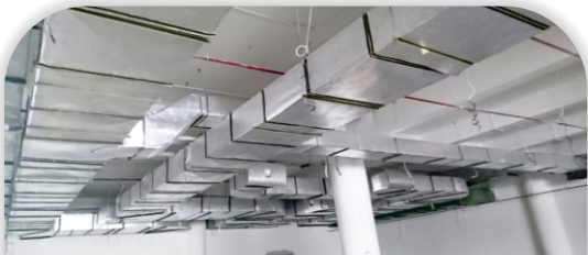
DUCTING AC DAN FRESH AIR
